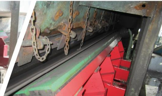
Power plant in Hubei
